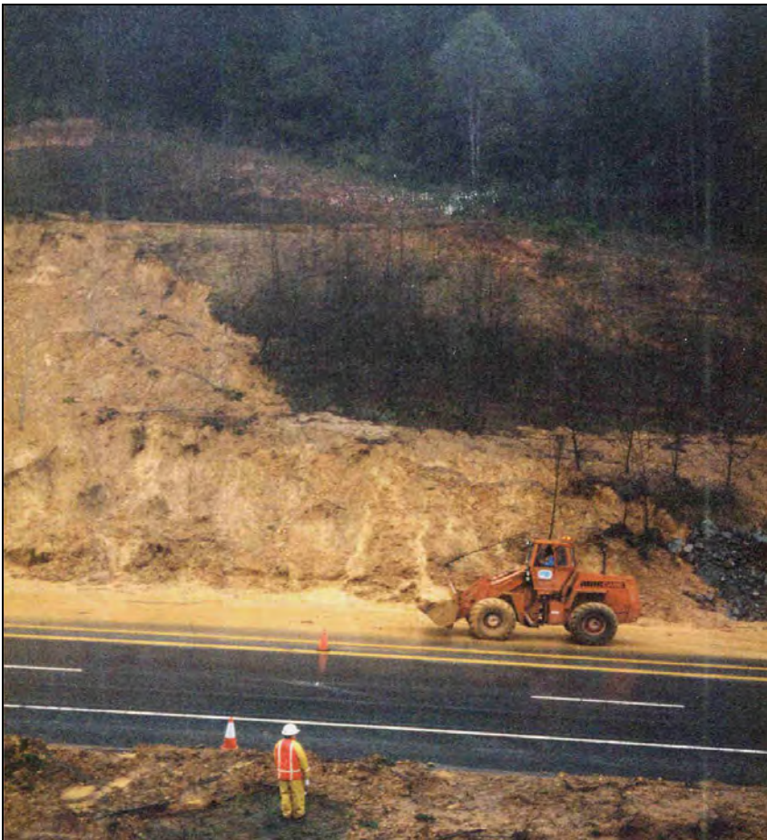
Figure 14-7. Highway 101 Landslide Clean Up, Winter 2005-06
